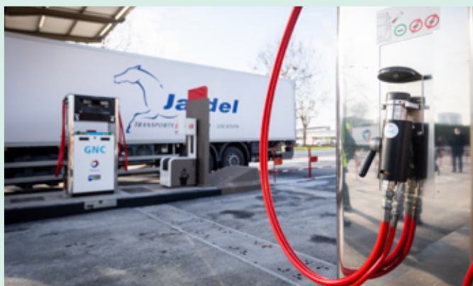
Station GNV - Gennevilliers, Hauts-de-Seine
